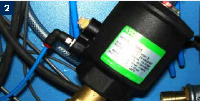
EN Solenoid valve on clean water supply.
